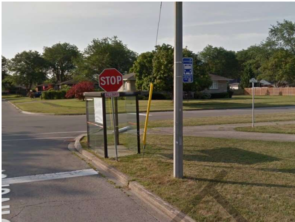
Figure 9: A non-accessible bus stop with a utility guide wire obstructing the landing area with reflective sheath.
