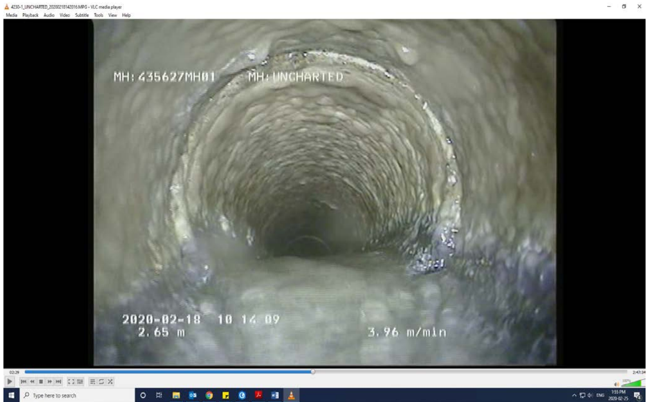
Picture 3: Michigan Street sewer in February 2020
