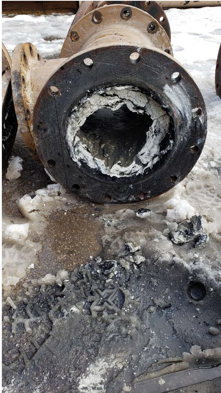
Picture 4: Dain City Sewage Pump Station – Piping replaced during Phase 2 of Forcemain replacement
